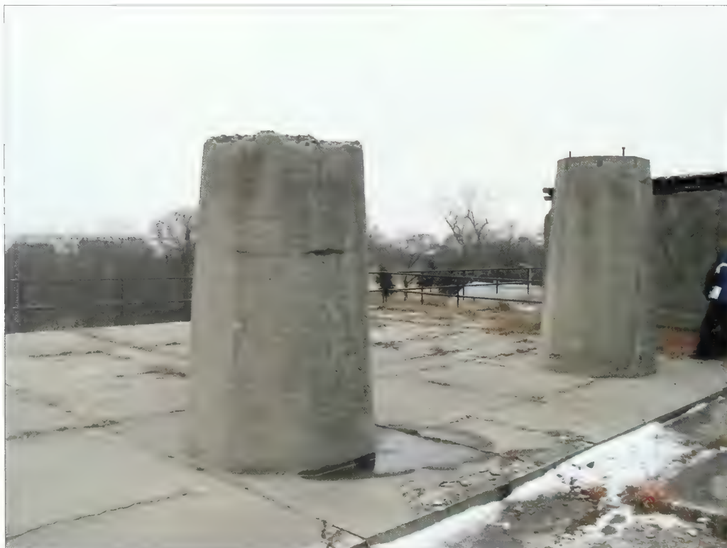
Figure 3.28. View looking northwest at concrete pillars, Battery Potter. South of the two groups of fire control stations, two concrete pillars remain from another structure that served as an additional fire control station (Olmsted Center, January 2009).
